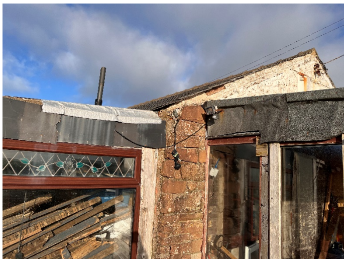
Poor quality extensions with thin walls and no potential for bats to take access to wall tops
